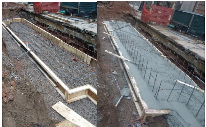
In Progress: the Installation of Seatwall B Formwork and concrete foundations on E. 25 th St. between Lexington Avenue and 3 rd Avenue
