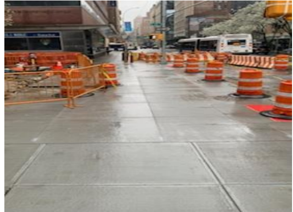
Newly reconstructed sidewalks/curb extensions on Lexington Ave. and E. 25 th St. looking Southwest.
