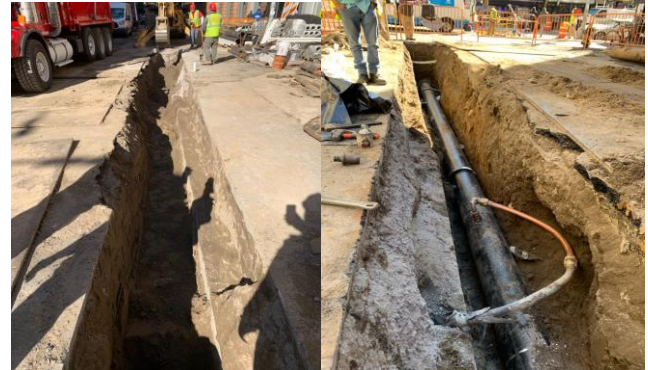
Newly installed 12” water main on E. 25 th St. between Lexington Ave. to 3 rd Ave. looking east.
