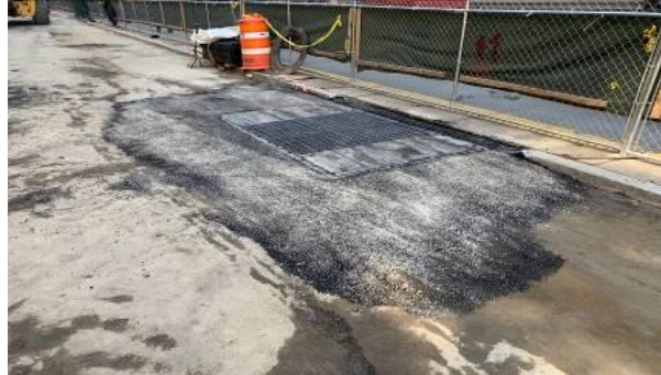
Newly installed electrical service box on E. 25 th St. bt Lexington Ave. and 3 rd Ave.
