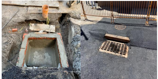
Newly installed catch basin on the N/W/C of E. 25 th St. and 3 rd Ave.
