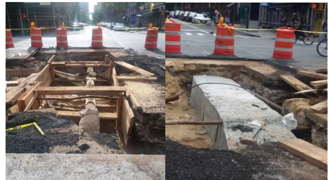
Steam main abatement and concrete encasement on E.25 th Street and 3 rd Ave. looking east.
