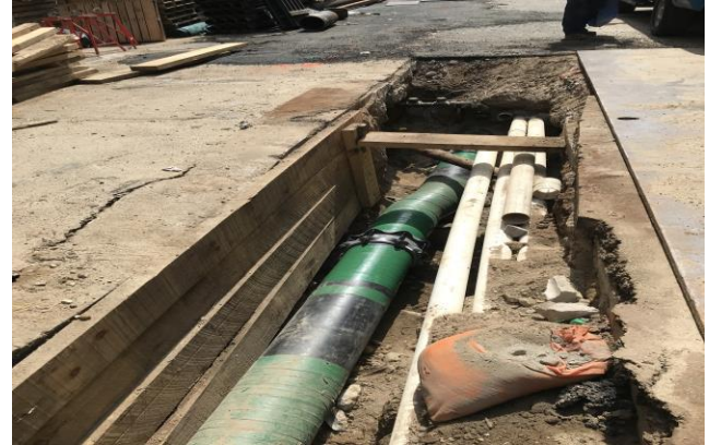
Newly installed gas main on E. 25 th St. bt Lexington Ave. and 3 rd Ave.
